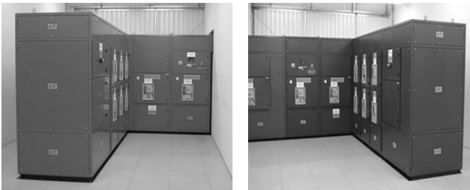
Figure 11 Datacentre with ACBs/MCCBs
